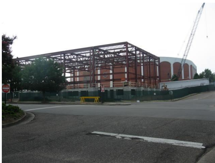
Figure 9 Example for a building constructed using steel – New Construction near Coliseum at MSU
